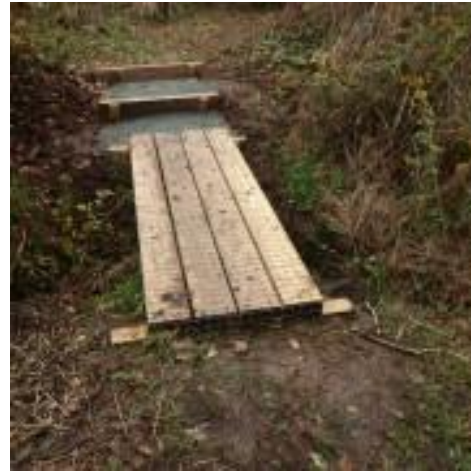
Simple bridge installed by trainees at Castle Bromwich Parkland. Source: Castle Bromwich Historic Gardens Trust
